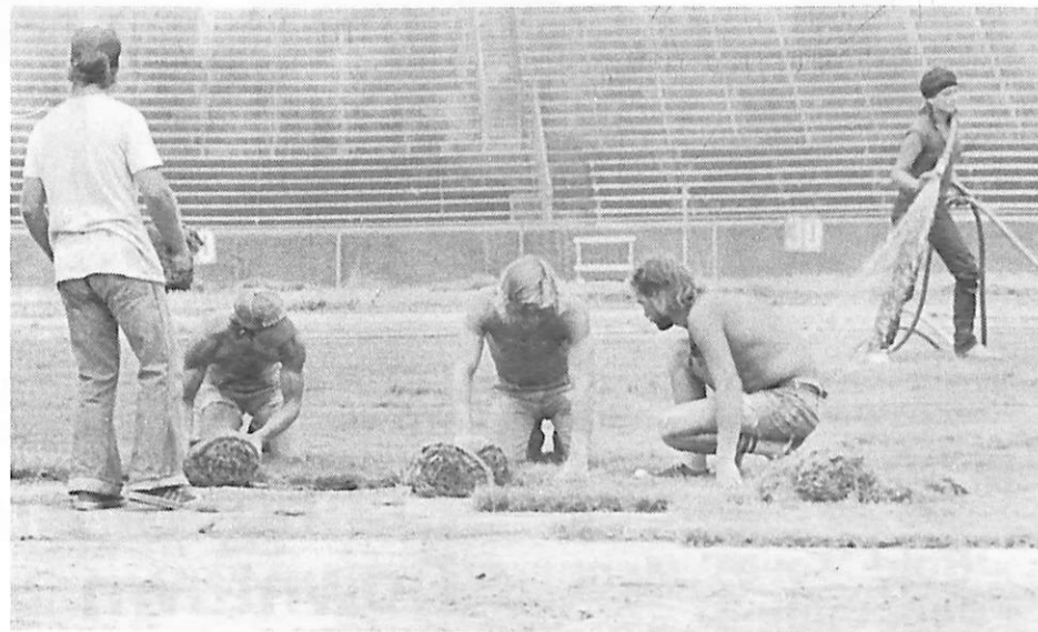
The Green Green Grass of Home: Hale Stadium under went a major transformation during the summer as an underground watering system was installed and new sod was laid over the entire football field.
