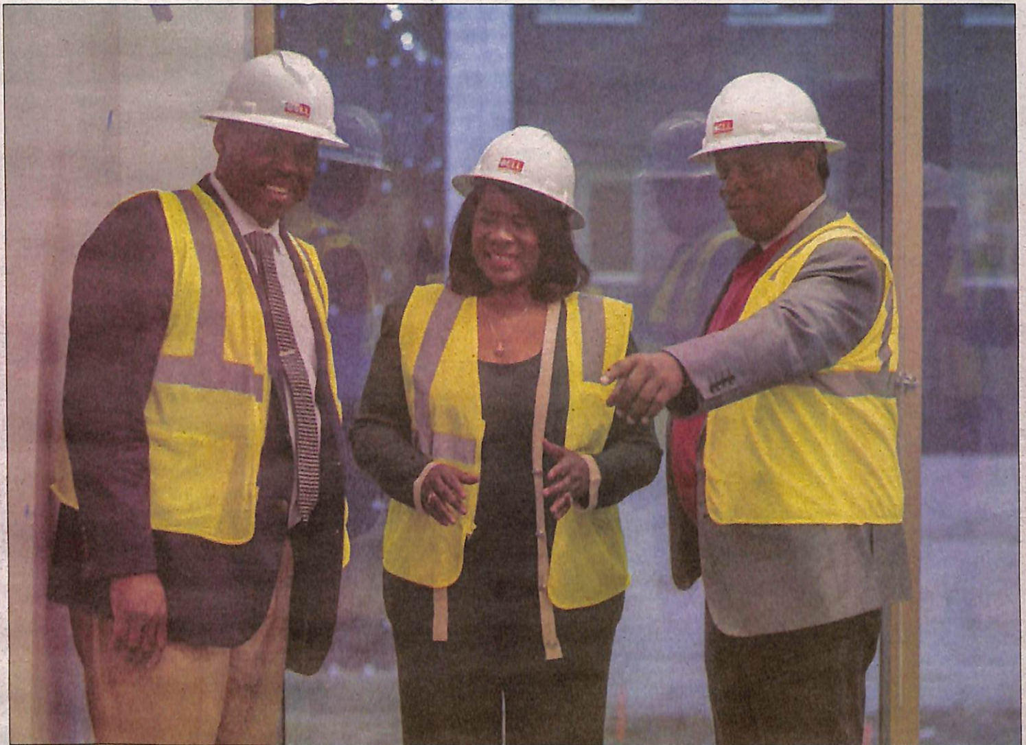
TSU President Glenda Glover tours residence hall construction site with Frank Stevenson, associate vice president for student affairs (left) and Dr. Curtis Johnson, chief of staff (right).
